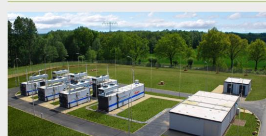
This power-to-gas plant, built by Eon in northern Germany, converts excess wind power to hydrogen and then injects it into the network system.
